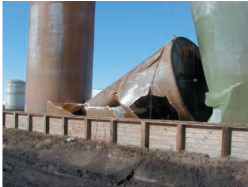
A combination of fill levels and weather conditions can lead to costly fiberglass tank collapses.
